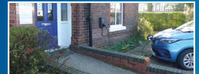
A charging point has been installed at the RNS office in Brigg.
